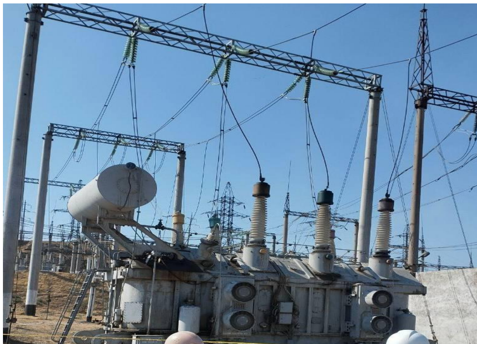
Figure 2. A 125 MVA transformer with a voltage of 220 kV at the Khakan substation in Andijan region.
