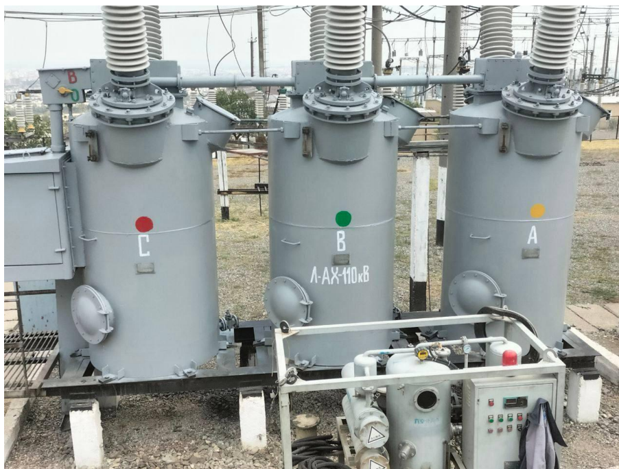
Figure 1. Oil fire extinguisher and related devices.
